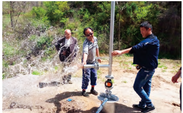
■ In Shanxi, we help improve the infrastructure and safe drinking water supply for local villagers
