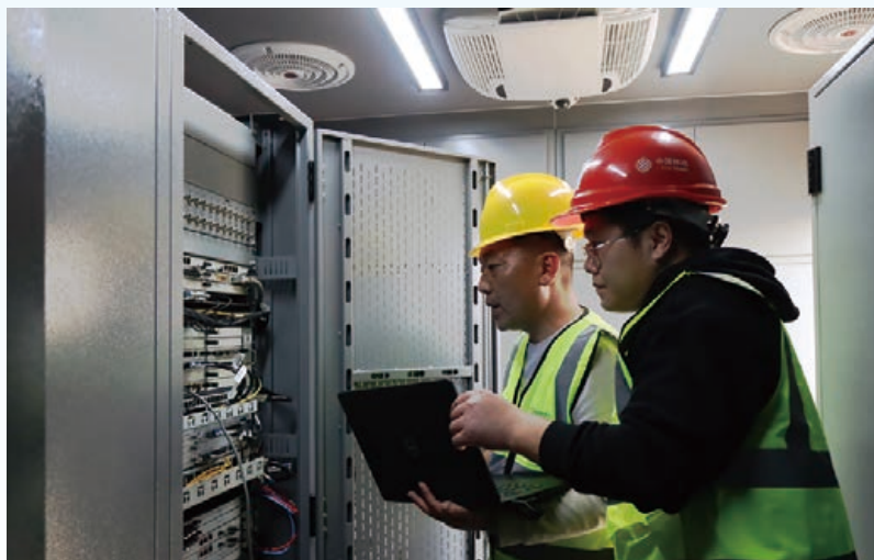
Staff conducted maintenance on intelligent city equipment
